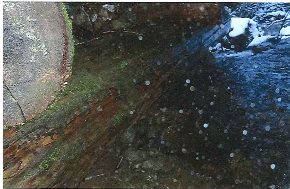
CK2003 Left Abutment Scour
